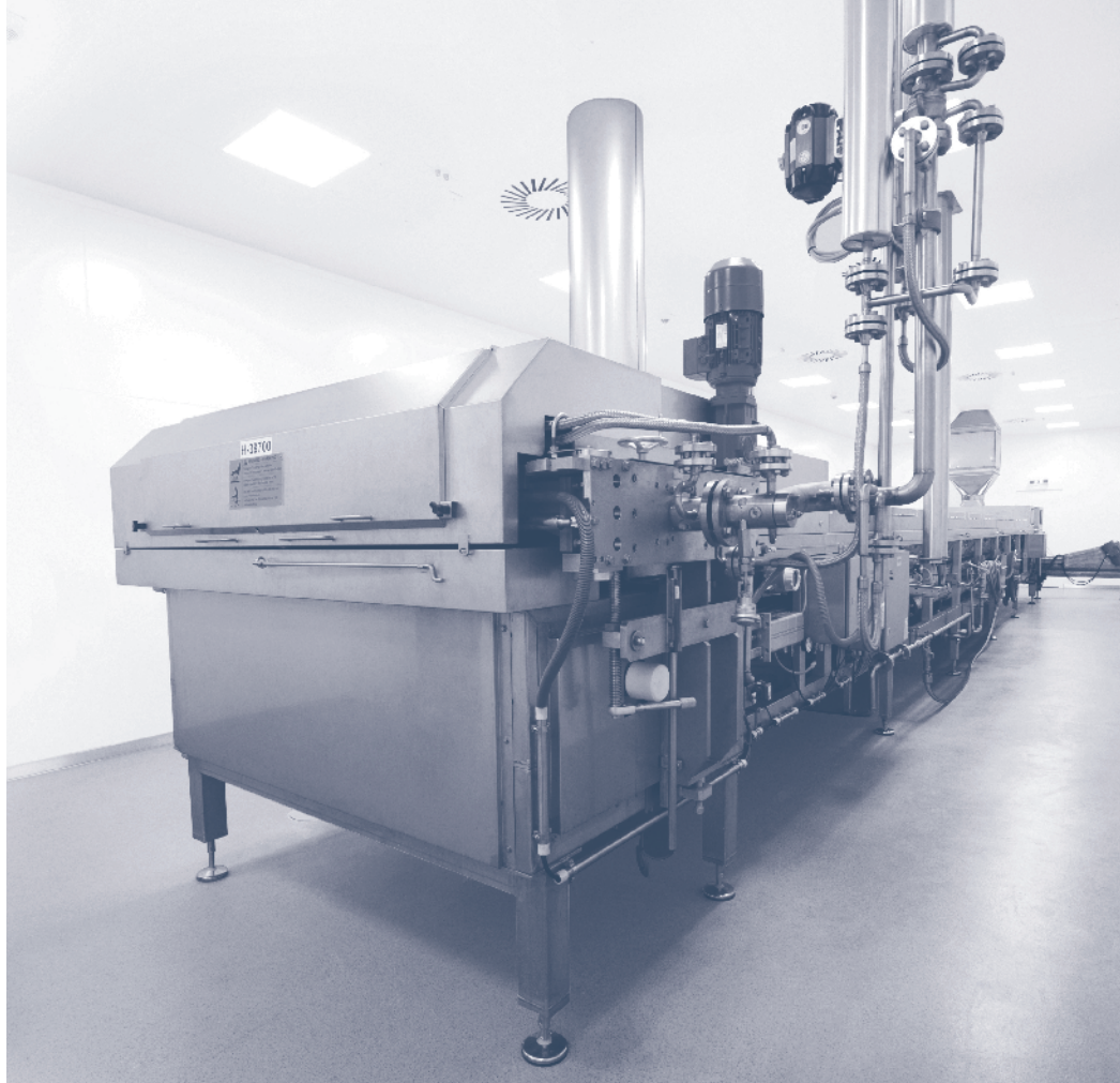
Rotoform installation in clean room.
